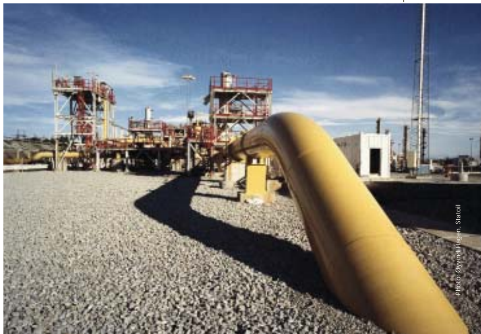
Pipelines at the Kårstø facility in Norway.
